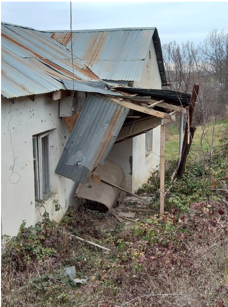
Image 2 . Damaged community building in Parukh village
